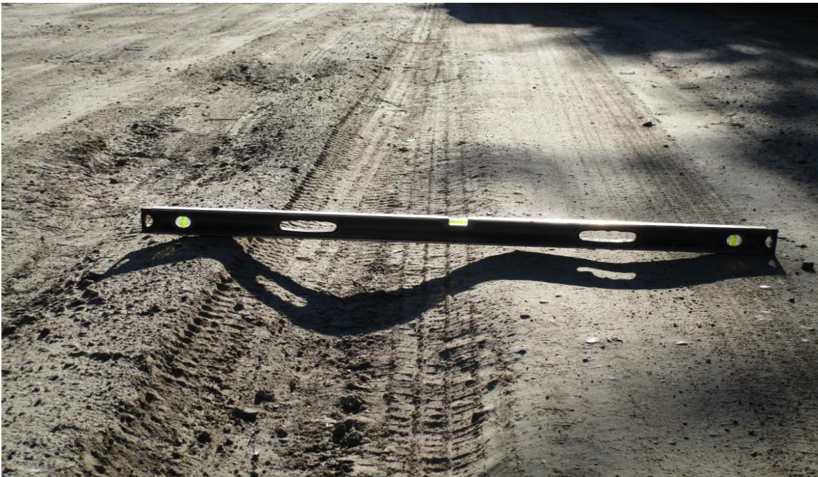
Boom Camp Road: Rutting, Washboard and Loose Gravel
