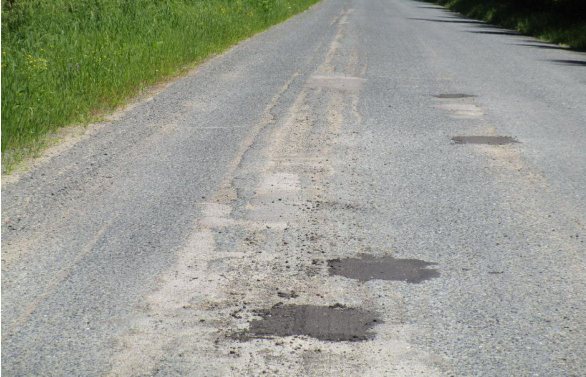
Pine Drive: Distortion, Ravelling and Cover Aggregate Loss
