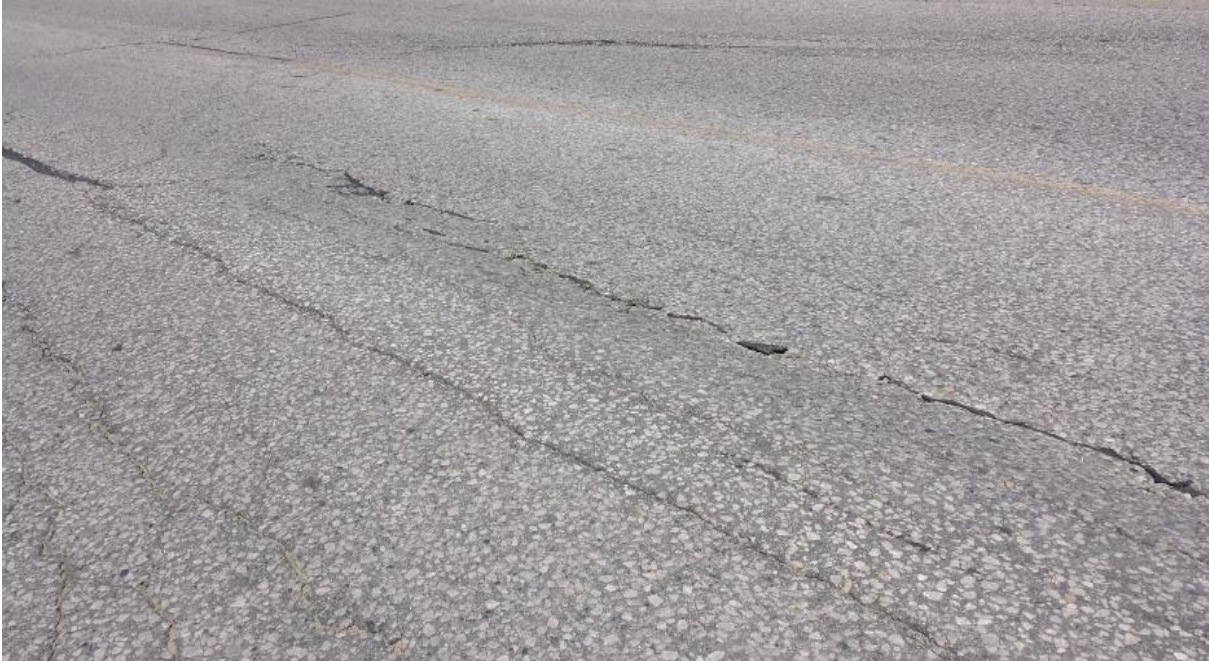
Robb Road: Rutting, Map Cracking and Longitudinal Cracking
