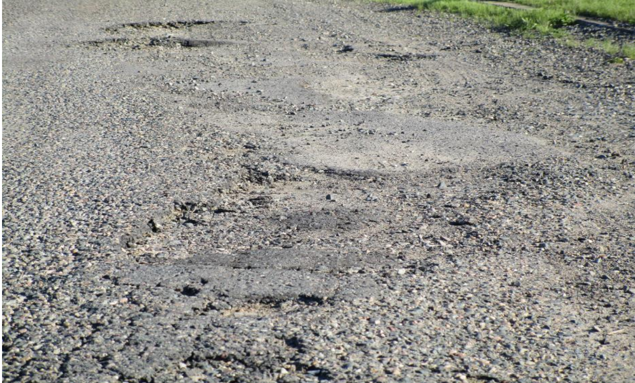
Marina Road: Distortion, Pavement Edge Cracking and Cover Aggregate Loss
