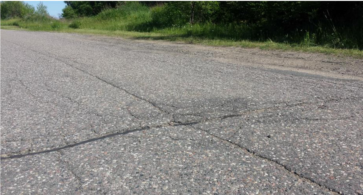
Birch Street: Ravelling, Longitudinal and Transverse Cracking
