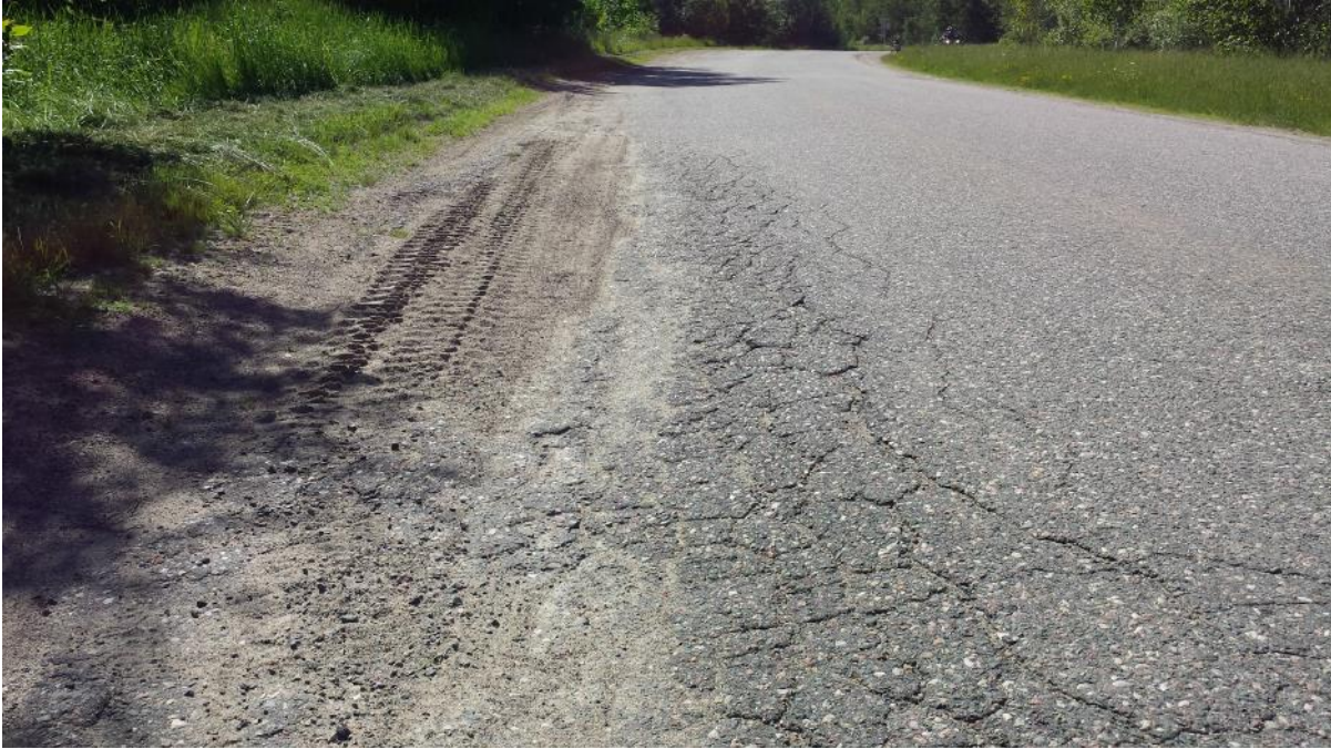
Schurm Avenue: Pavement Edge Alligator Cracking
