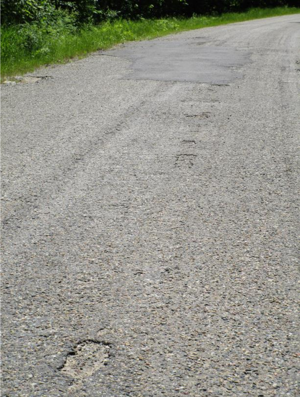
Old Steel Road: Ravelling and Cover Aggregate Loss
