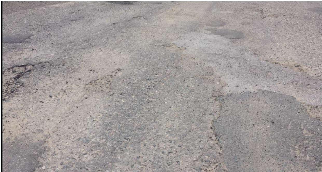
Magog Lake Road: Distortion, Ravelling and Center Line Cracking
