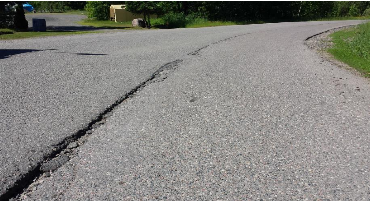
Robb Road: Severe Center Line Cracking
